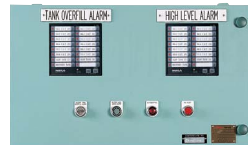
HIGH AND OVERFILL ALARM PANEL
