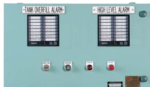
HIGH AND OVERFIRL ALARM PANEL
