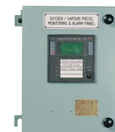
MONITORING & ALARM PANEL
